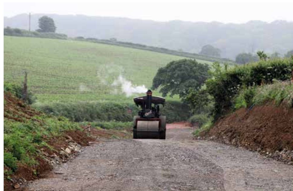
The new access road at Prospidnick is quite steep where it leaves the local lane and, in fact, climbs all the way to the station yard. This made for some interesting driving for Josh as well as some lovely sounds as the Burrell made its way very slowly up the incline before quietly reversing back down again.
