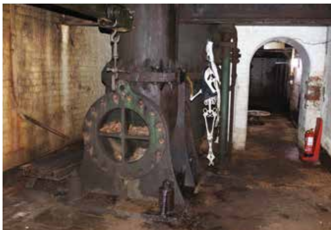
Down at the bottom are the sewage pumps. A large sewage main still runs below the floor.
