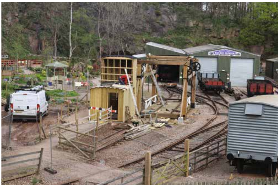
A general view of the site with the lift bridge and its control cabin in the centre, still under construction. The railway museum is to the right with the standard gauge running shed alongside. The garden and narrow gauge railway are to the left.
