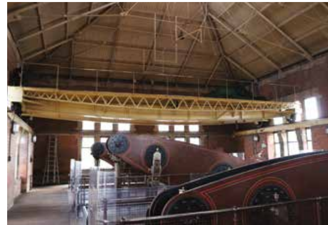
Three of the four beams at the top of the engine house. The travelling crane used for maintenance is also visible.
