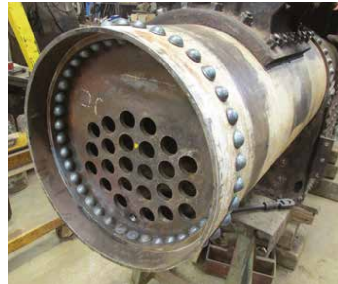
A month later and the front tubeplate has been rivetted in place.
